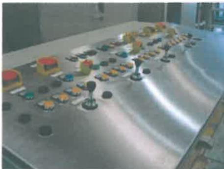
Main Control Pulpit
